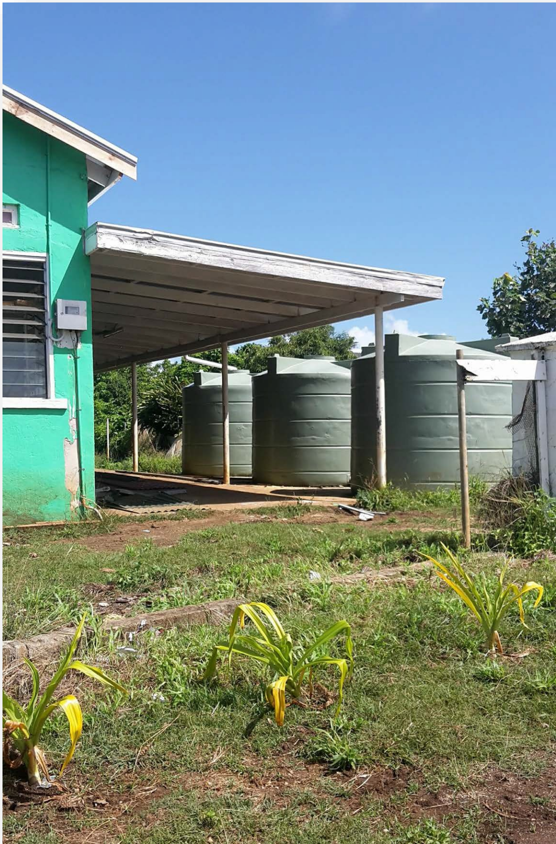
Figure 4.5. A community hall on Ha'apai that was retrofitted with water tanks following TC Ian. Source: Authors own, 2017.
