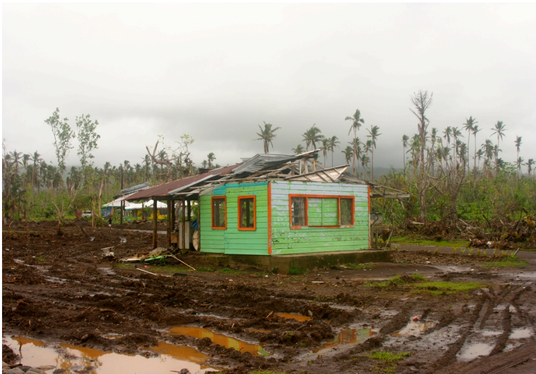
Figure 1.1: Housing damage following cyclone Evan
